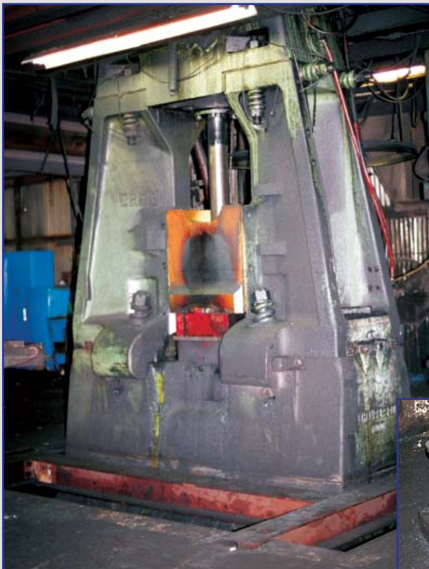
CECO #23 installed on FSV20-164-6S Viscous Damped Spring Mounts.
